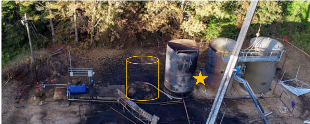
Figure 3. This post-incident photo shows the location of the welding activity that triggered the explosion (gold star) and the pre-incident location of the fourth tank, which was launched by the blast and propelled into the woods shown in the background. (Credit: Red Hancock with annotations by CSB)
