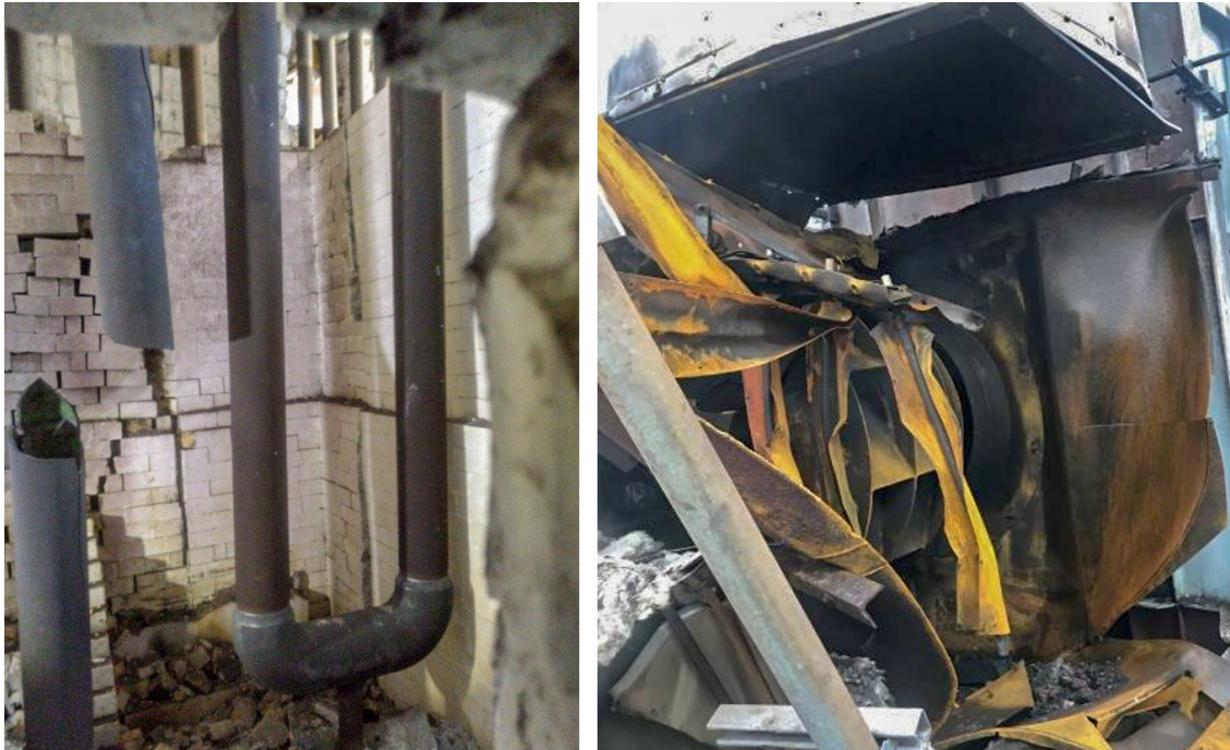
Figure 5. Fired heater explosion damage. The left image shows the broken tube and walls, and the right image shows a fan. (Credit: Chevron Phillips)
