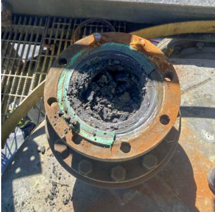
Figure 2. Solids in the rupture disc inlet piping. (Credit: Tronox)
