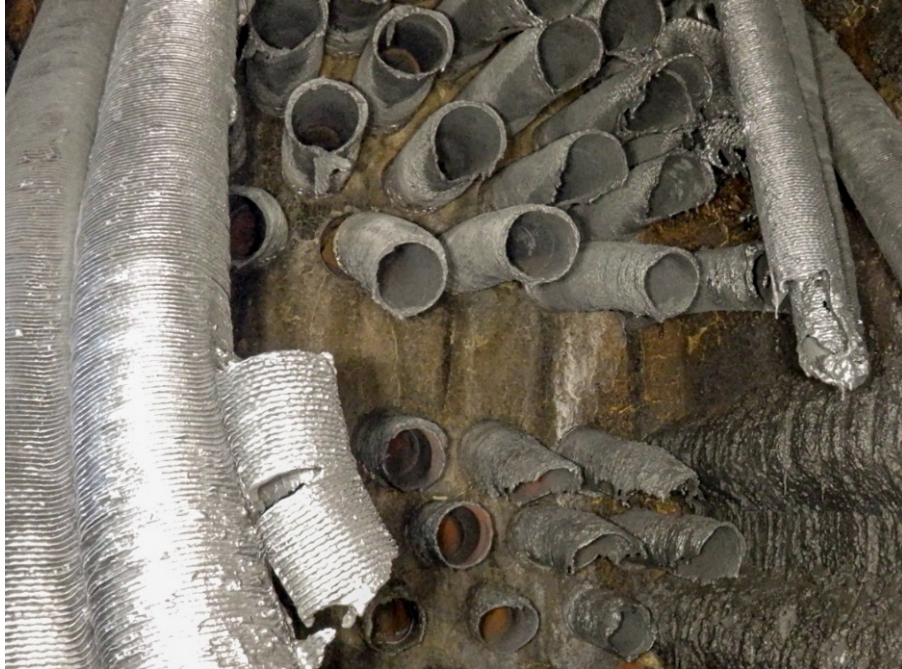
Figure 19. Broken fired heater tubes. (Credit: LyondellBasell)
