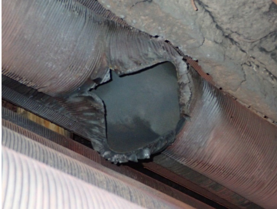
Figure 7. Ruptured fired heater tubing. (Credit: Valero)
