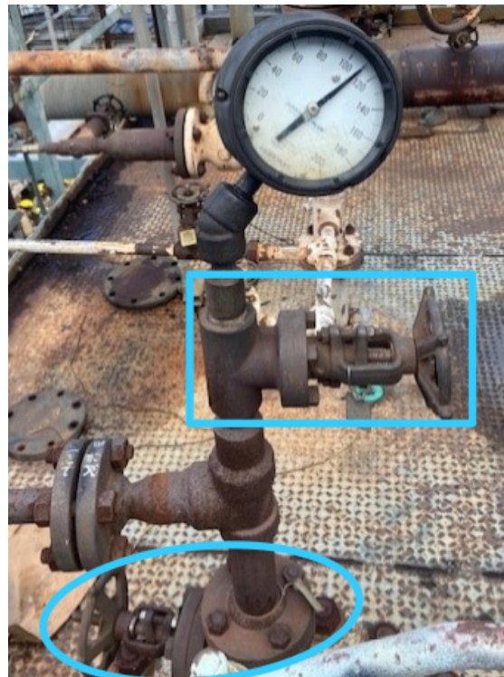
Figure 1. Photo of the pressure gauge and valves involved in the incident. (Credit: Marathon, annotations by CSB)
