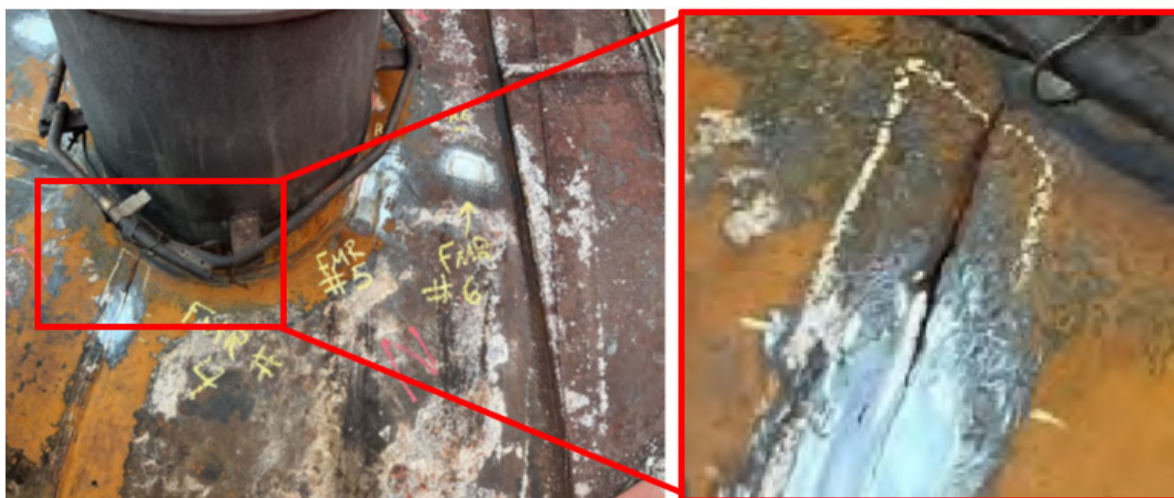
Figure 2. One of the cracks in the reactor’s head. (Credit: LyondellBasell, edited by the CSB)
