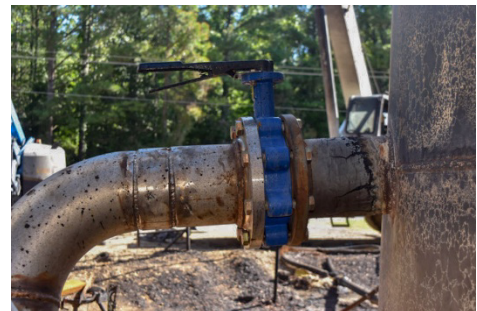
Figure 2. Open valve between new piping (left) and an old tank (right). (Credit: Red Hancock)
