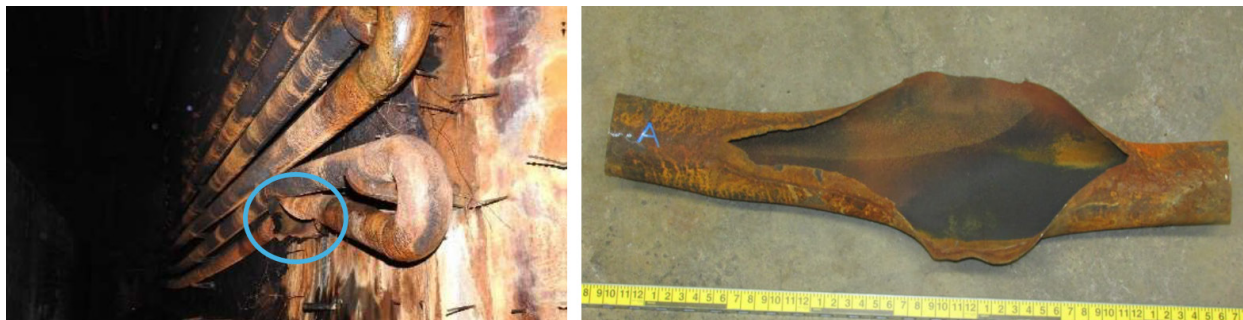
Figure 9. The ruptured tube within the fired heater (left) and after removal (right). (Credit: Delek)
