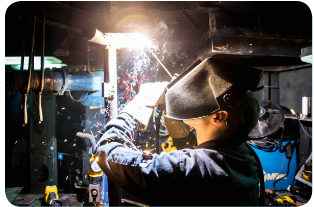
Follow safety standards to prevent common hazards and maintain a safe jobsite.
