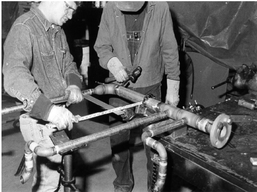
Figure 9.2 Weld fit-up and gap examples. (Photograph courtesy of TEAM Industries, Inc., Kaukauna, WI.)
