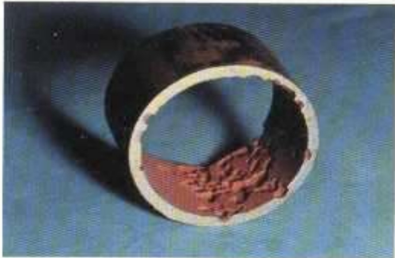
Economizer tube severely damaged by oxygen.
