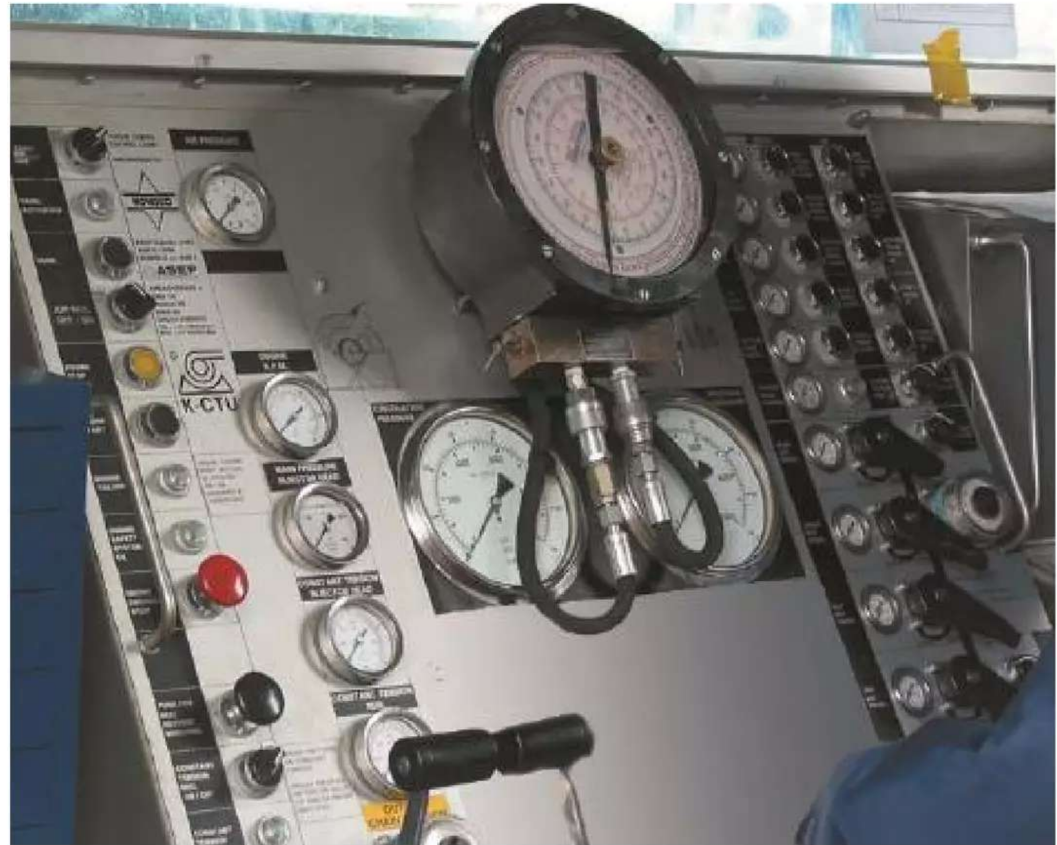
OVERVIEW OF ALL CONTROLS/GAUGES
